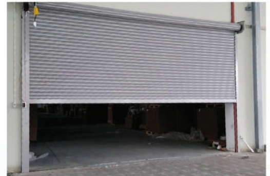
Automatic rolling shutters
